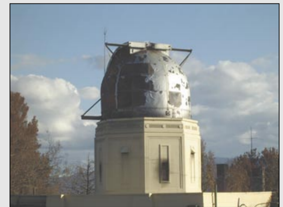
The Heliostat dome after the firestorm of 18 January 2003
