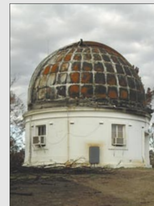
The Reynolds dome after the 18 January 2003 firestorm
